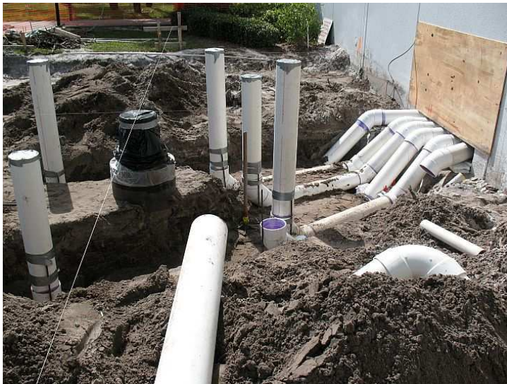
Fig. 4: Site excavation before pouring the vault foundation. The top of the source well is clearly visible to the left of image center. The PVC piping provides cable raceways between the vault and the Intersil Palm Bay building 58 control room (right).
