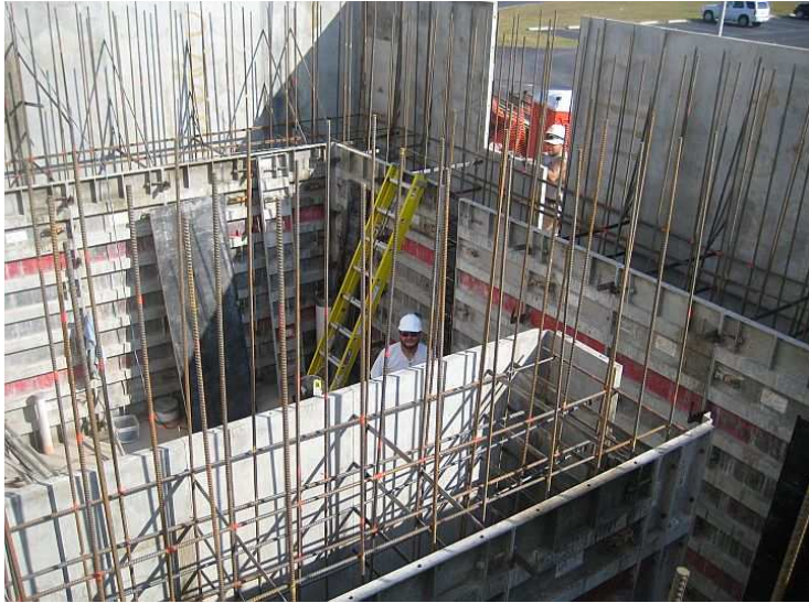
Fig. 5: View of wall forms before the second (wall) concrete pour. The labyrinth vault access architecture can be clearly seen.
